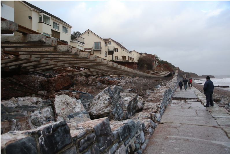
Figure 5.4. Photo showing damage to the retaining wall bounding the mainline railway at Dawlish (©Matt Clark, Met Office).
