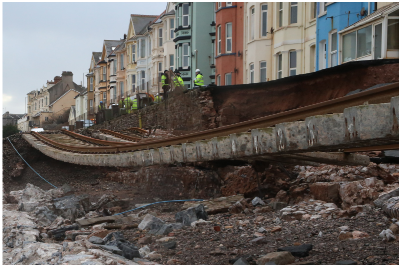
Figure 5.3. Damage to the Southwest mainline railway at Dawlish (Devon) after the storm of 4–5th February. Breach of sea defences and destruction of retaining wall, left rails suspended in mid-air after foundations were washed away (©Matt Clark, Met Office).
