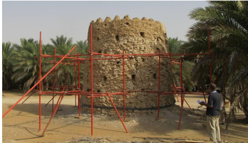
Figure 8: Hayla Tower in 2011 during installation of retaining straps. Source: photograph by author.
