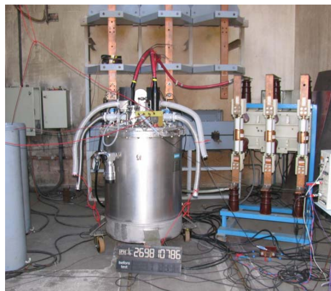
Figure 2. Fully assembled FCL module in the test cell of the IPH power testing lab in Berlin.
